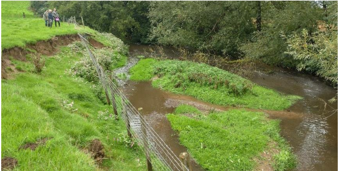
Fig 16. Another failure of the stock-proof fencing because it was placed too close to the top of the bank on an artificially straightened section and the river had undermined the whole lot. A deposition bar had formed within the channel. Note the lack of erosion on the LB afforded a native tree and herb flora in stark contrast to the grazed RB.
