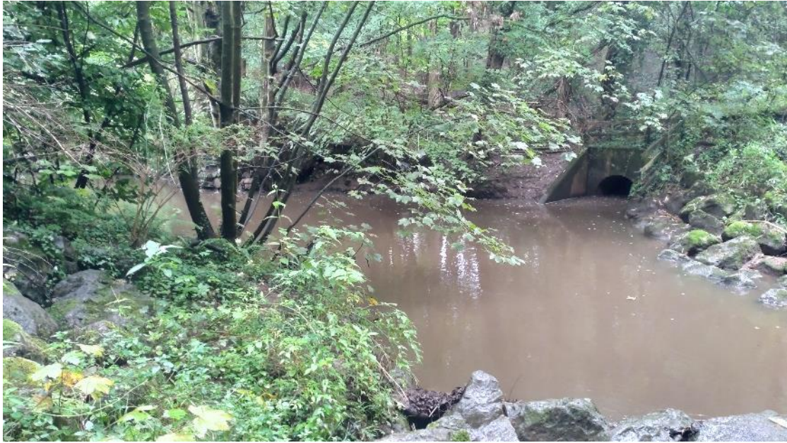
Fig 10. On the LB, u/s of the M6 flyover, a large culvert formalised the flow from a small beck network, seemingly converted to agricultural drains, and presumably with contributions from the motorway which will be a focal point for pollution.
