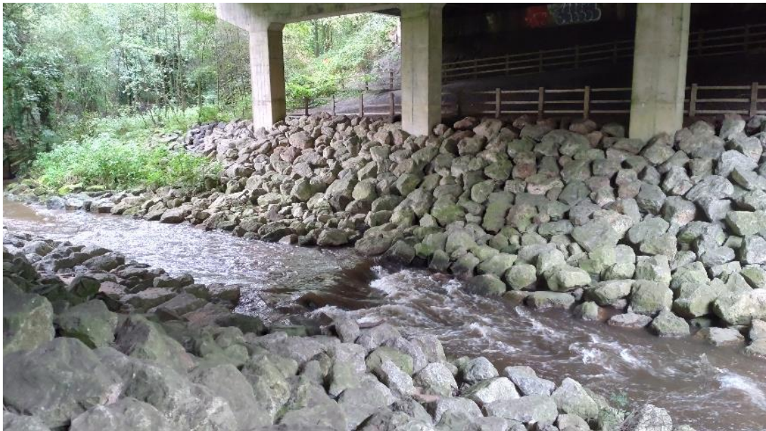
Fig 11. Large boulder revetment underneath the M6 flyover, pinching and straightening the channel, and increasing flow velocity for the span of the bridge.
