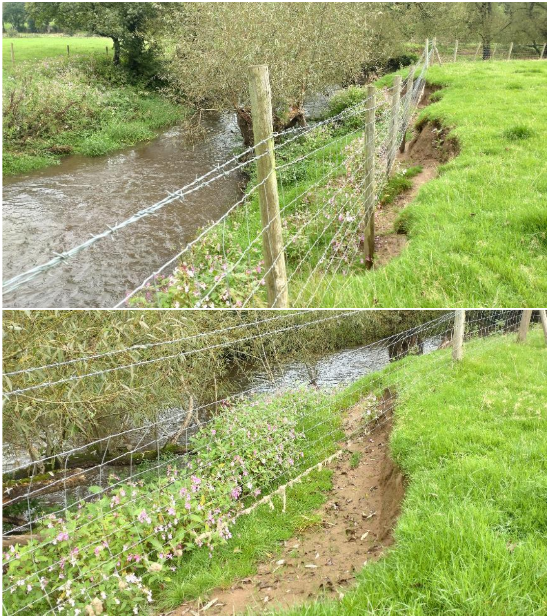
Fig 17. More slumping of the bank where the fence has been placed too close to the top. Sheep were clearly exacerbating these scallops to gain access under the fence, maintaining the area as bare soil and hence increasing the risk of further erosion under spate flow. There was no discernible difference in sward height on either side of the fence, indicating that sheep had unfettered access.
