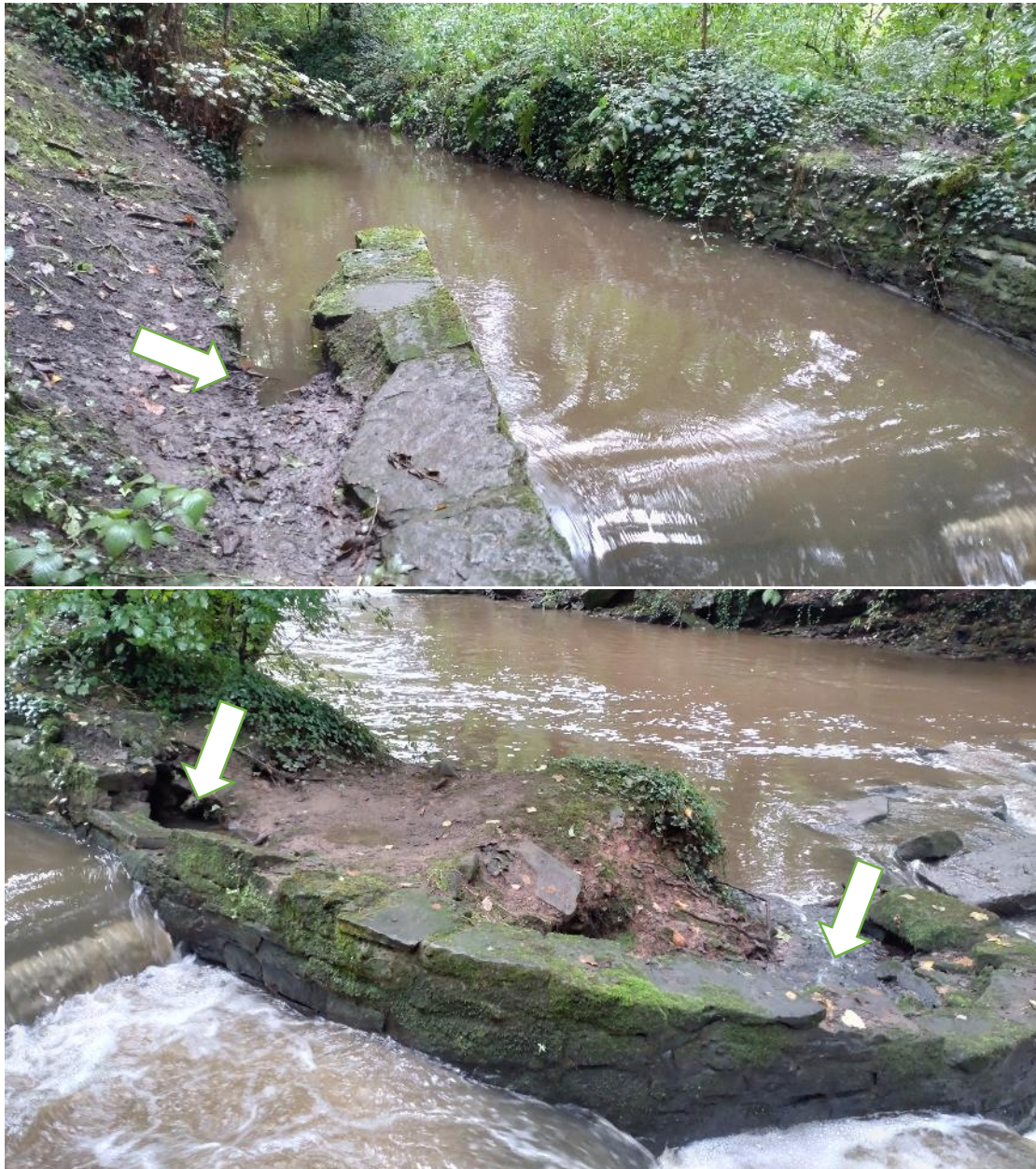
Fig 6. Erosion detail around the fish pass. Clearly time and expense has gone into the building of this structure, yet it was in a poor state of repair and likely to fail in the near future without a little further investment.
