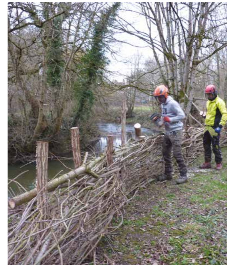
Left: Putting the finishing touches to the dead hedge in Rodden Meadow. Right: Before and after building the dead hedge, showing the heavy banktop erosion (and thus siltation) that it’s designed to protect against
