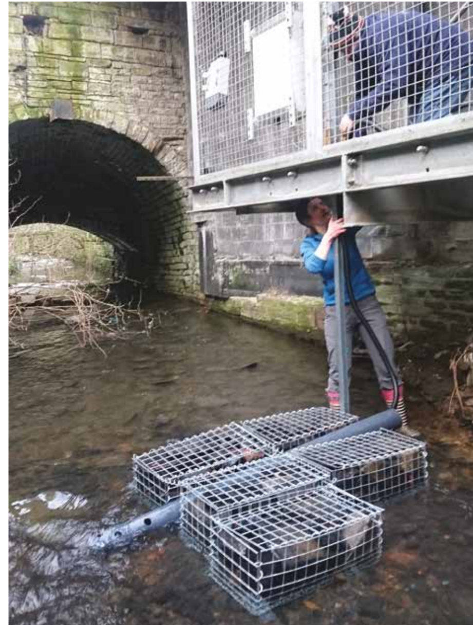
Setting up a WaterBox water quality monitoring sonde in Bradford: the very first to be installed outside Taiwan
