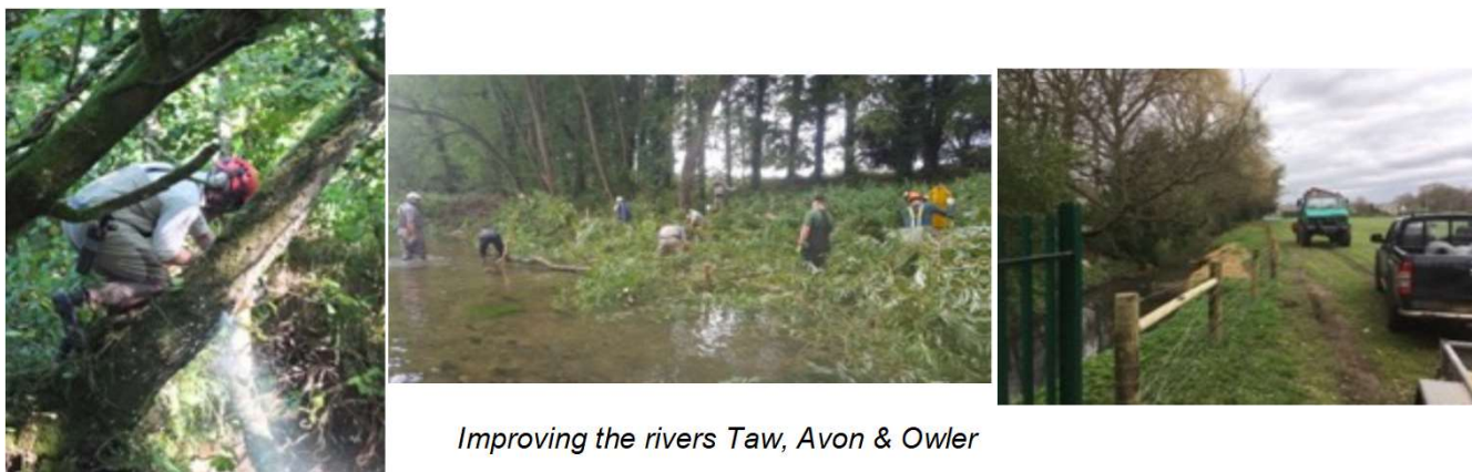
River Dove: ponded upstream (above left); weir removed (above middle) and river released (right).
