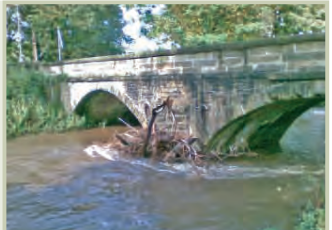
...JUST UPSTREAM OF BRIDGE PARAPET ACCUMULATING UNSECURED, NATURALLY-OCCURRING LWD
