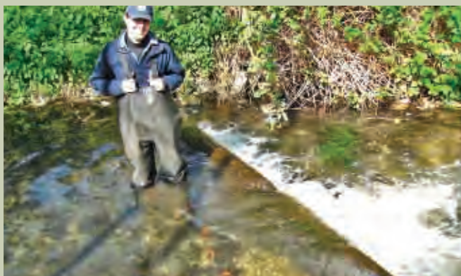
SMALL WEIR ON RIVER WANDLE BEFORE REMOVAL OF TOP COURSES OF STONE
