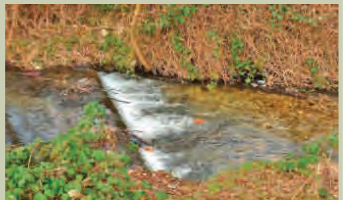
THE SAME WEIR AFTER THE REMOVAL OF TOP COURSES OF STONE. NOTE GRAVEL RAMP THROWN UP BELOW THE LOWERED WEIR
