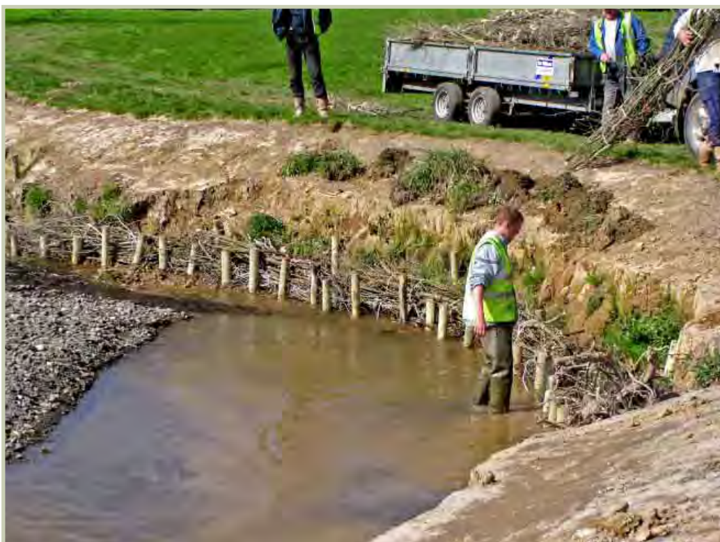
LIVE WILLOW BUNDLES BEING INSTALLED TO REDUCE EROSION ON OUTSIDE OF BEND
