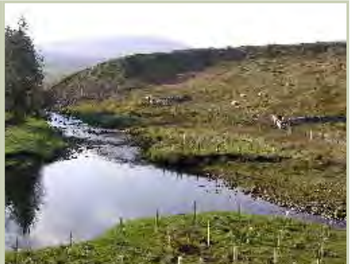
THE SAME SECTION OF RIVER AFTER COMPLETION OF THE WORKS- MARCH 2007. NOTE NEW FENCING, TREE PLANTING, AND VEGETATION GROWTH ON PREVIOUSLY BARE BANK
