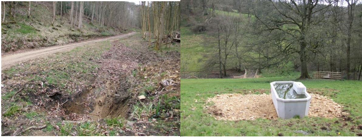
Forest tracks diverted into soakaways and spring-fed drinking troughs to keep livestock out of watercourse
