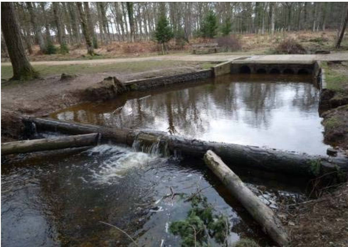
Fig.(11) A K dam on the Bratley Water (Lymington) constructed to help ease fish through an ‘Irish ford’.
