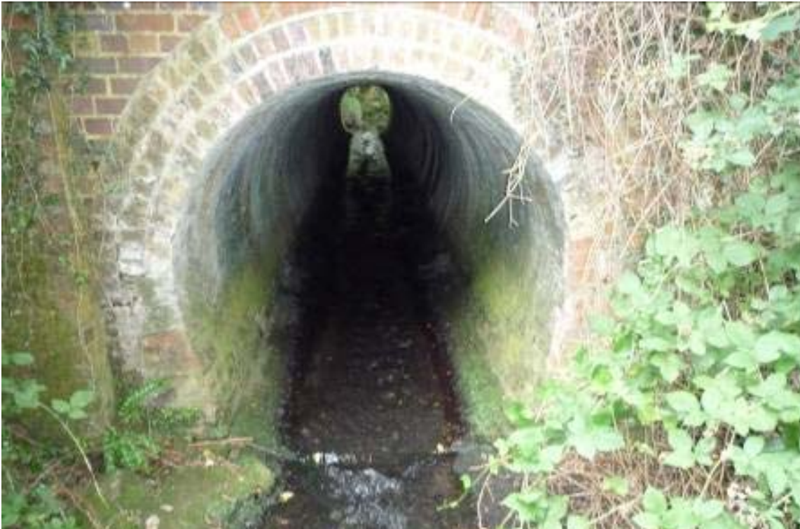
Fig.(19) A culvert on the Plumpton Mill Stream is a priority on the Ouse
