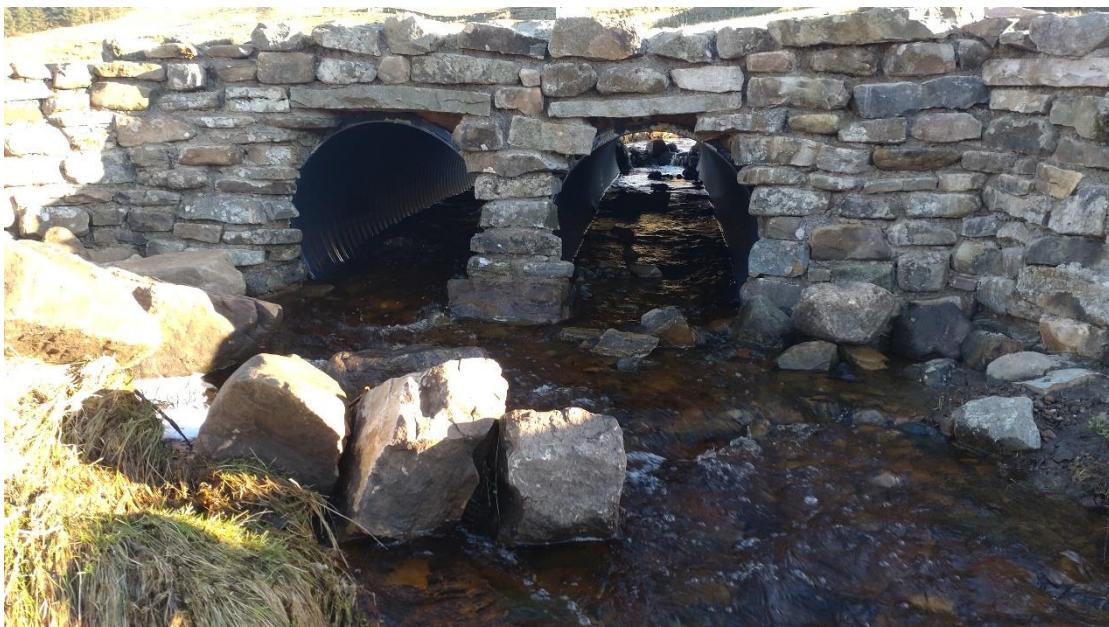
Fig 14b. Twin culvert pipes discussed on site. On the d/s side looking u/s, it was evident that the pipes had been buried to a certain degree and the angle of slope sufficiently low to retain bed substrate. A watching brief is required for potential development of scour below the pipes which could lead to bed lowering and perching of those pipes.
