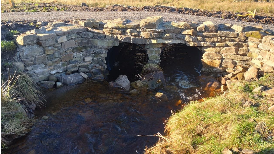
Fig 14a. Twin culvert pipes discussed on site. On the u/s side, there was already evidence of deposition of larger boulders (esp. at left-hand pipe) under high spate flow when the capacity of the pipes would have been exceeded and water had backed-up. These created a perch at the u/s side, visible as the cascade of water into the right-hand pipe. Ongoing maintenance issue.
