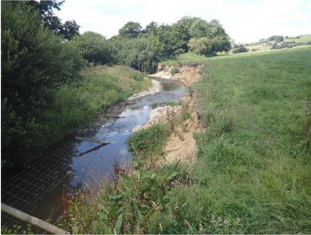
Photo 18: Insufficient buffer, erosion has taken place before the bank has stabilised or been strengthened through tree roots. Fences should be set well back from the river, 5 metres at a minimum.
