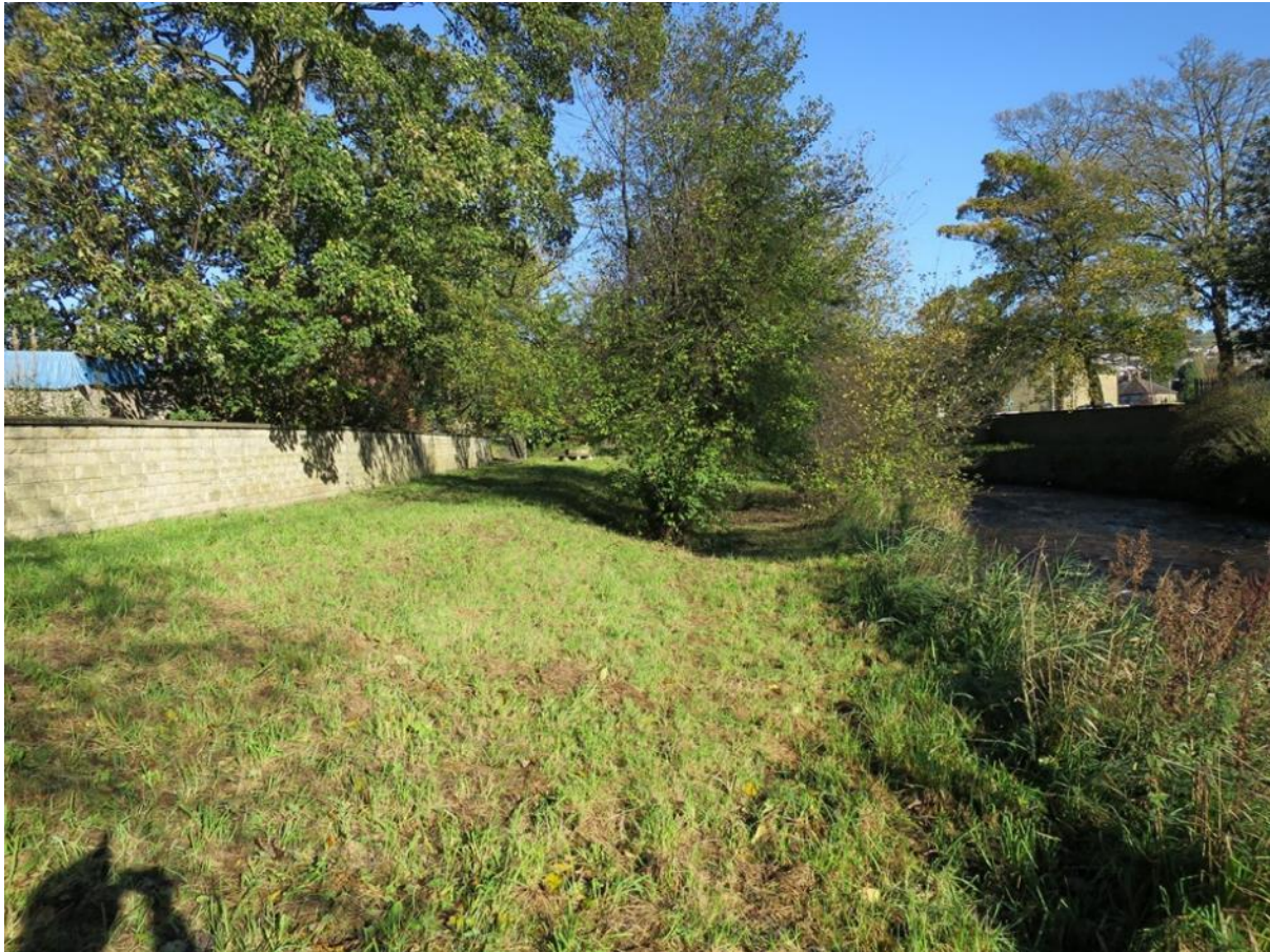
Figure 12: Grassed area enjoyed by local walkers with flood defence wall to the left of the frame and unmown buffer strip to the right. The opportunity for at least some natural over-land flow during spate conditions (and the refuge habitat created by the unmown buffer strip) are ecologically valuable features that should be preserved. The extent and value of the buffer vegetation could be extended by encouraging the wildflower seedbank for a greater proportion of the bank (with a mown ride/path maintained for walkers).
