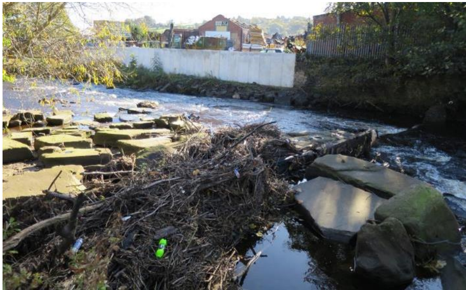
Figure 16: The wooden boards indicate the previous height of the weir crest. Note the brash accumulation at what was previously the entrance to the rock-ramp fish pass on the LB (left of frame).
