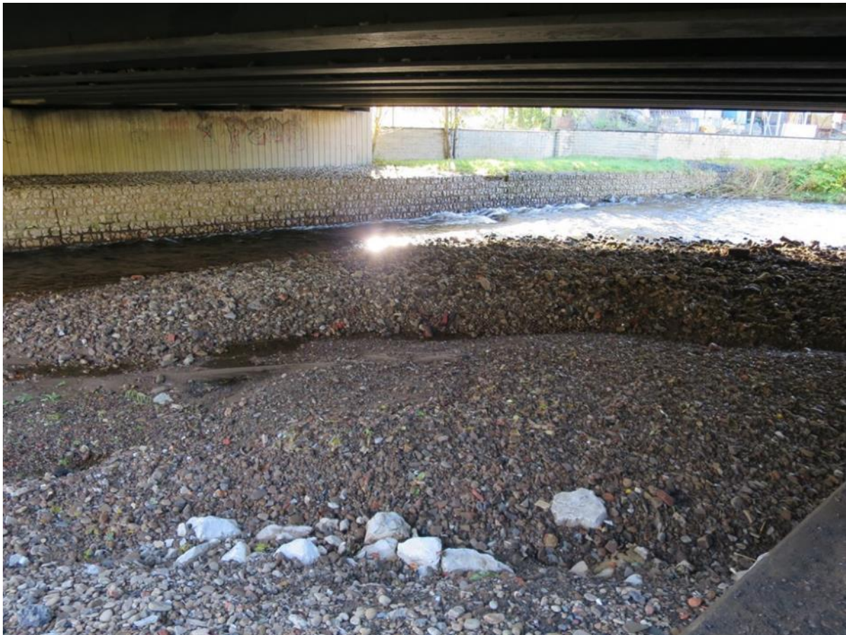
Figure 13: Recent dredging has been replaced with gravel and cobbles under the A650 bridge. This is an inevitable consequence on a steep, rain-fed river. As well as the position on a bend (where deposition is favoured on the inside of that bend) it is common to find that the riverbed beneath large bridges has been levelled artificially. This produces a break in the natural longitudinal bed-slope of the river – and the flat “pan” which results acts as a natural sediment trap.
