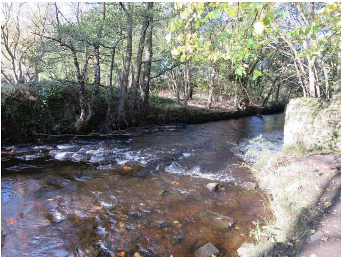
Figure 27: Probably the site of an old weir structure that has degraded over time or been demolished in the past.
