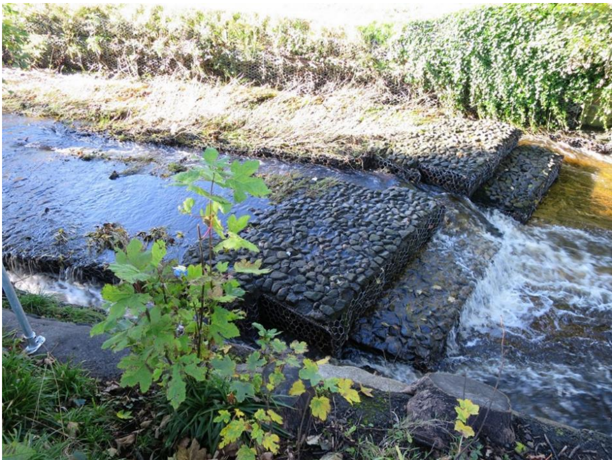
Figure 9: Modern (gabion) structure which splits low flows into three narrow channels (each impassable in an upstream direction by most fish under most conditions). The first of the three low flow channels one hugs the RB, one runs down the centre and one hugs the LB. All three discharge onto a shallow, smooth concrete apron that is impassable to fish. The gabion mesh is already beginning to degrade and will form a "gill net", a trapping hazard to aquatic life as the degradation progresses.
