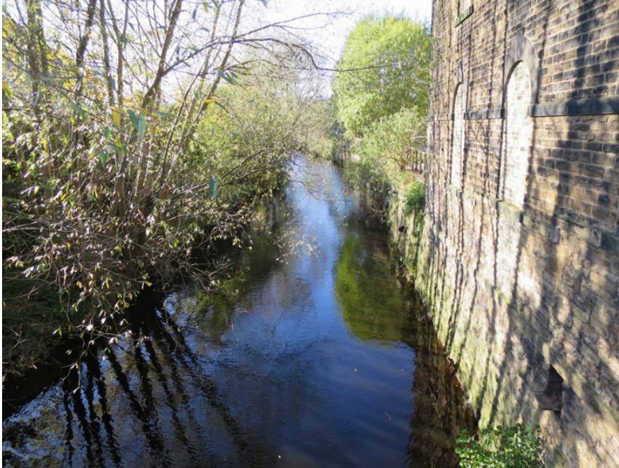
Figure 23: An extensive impounded reach photographed facing upstream at SE 06641 41169. Due to the overall high-gradient of the natural riverbed, a relatively large weir structure is probably responsible for such a large impounding impact.
