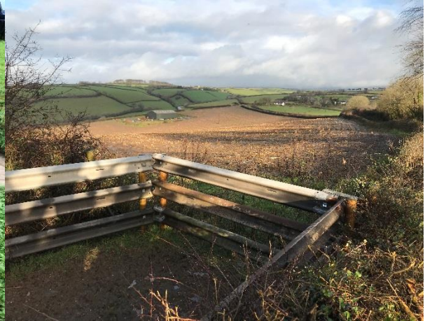
Field causing sediment pollution
