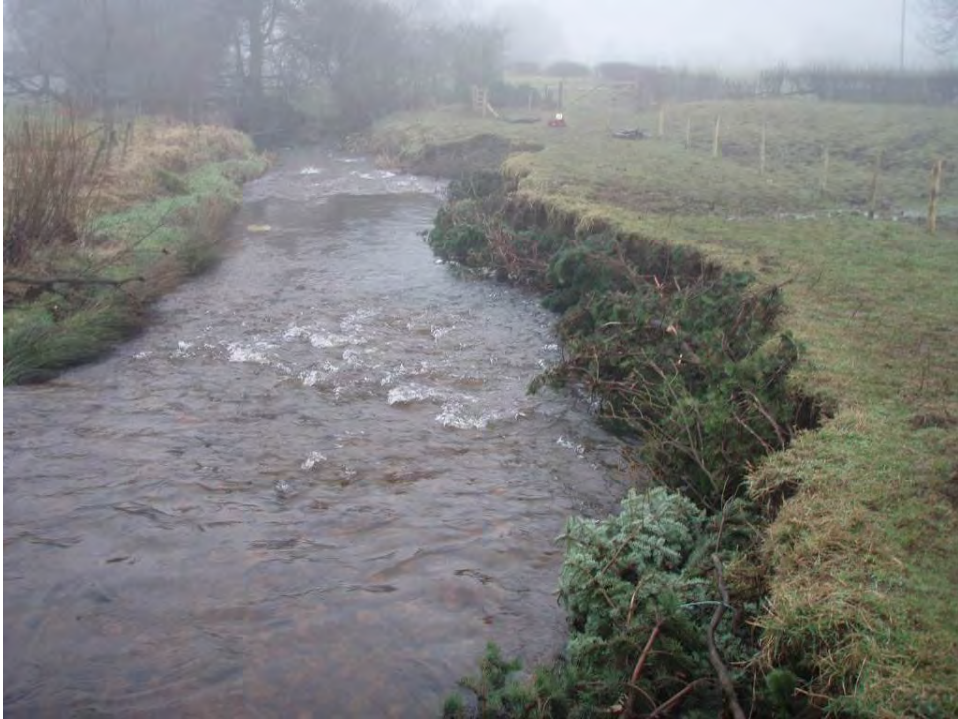
Photo 6 January 2009. View downstream towards footbridge and DCAC signing-in box at Ludburn Farm, immediately after installation of conifer brush at the toe of the bank and fencing well back from the river. (NGR SK0947562521).
