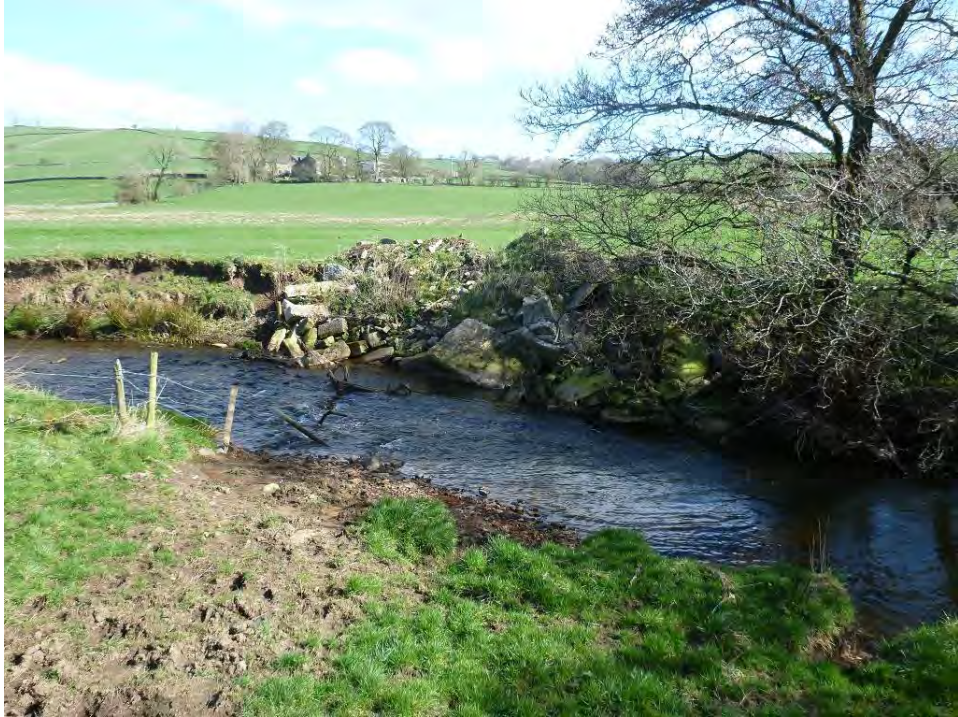
Photo 26 Hard bank protection such as this does not reduce the shear stress caused by fast water, hence erosion tends to occur where the stone begins and ends, undermining it. Use of brushwood and willow is preferable as it absorbs the energy of the water, binds the bank with roots and provides good cover and habitat.
