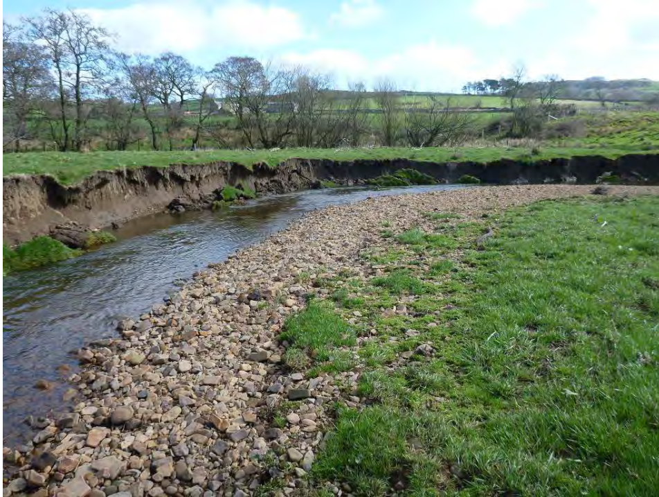
Photo 20 Rapidly eroding bank. Erosion may be slowed by stabilising the bank with brushwood and willow (see Photo 22), which would tend to focus the river energy into scouring the river bed and creating more depth; along with the woody cover, this would improve the fish holding capacity. Livestock exclusion would be ideal, but the use of thorn brushwood and willow may provide some grazing protection. Stopping bank erosion is not a possibility, nor desirable, but slowing it to improve habitat is.
