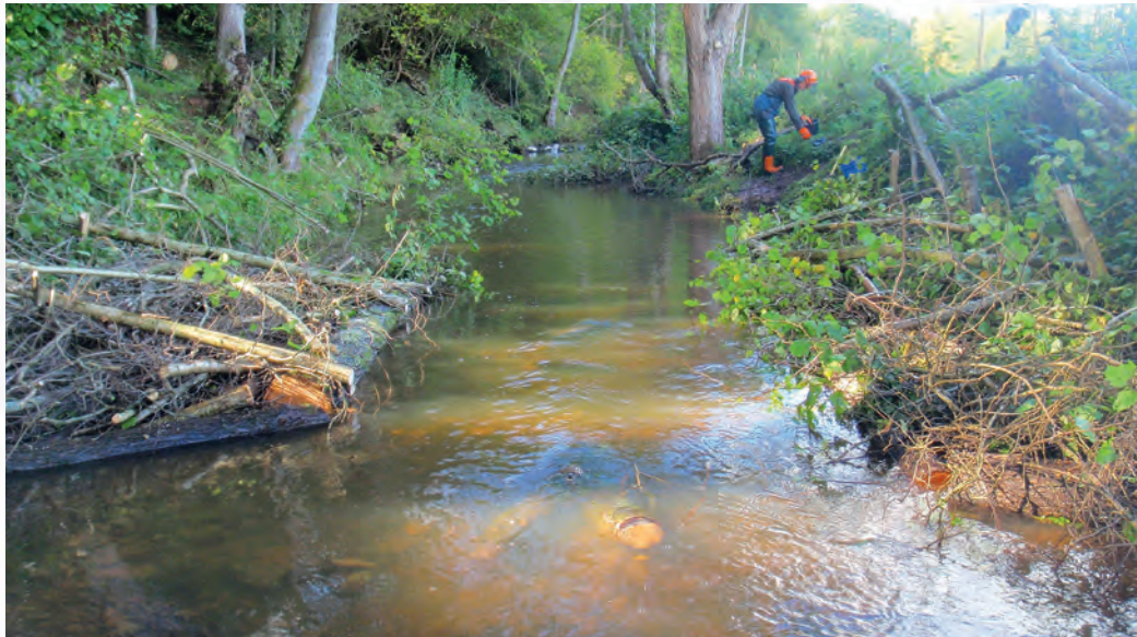
Pinch point on the Dulas brook. Note Y-shaped log and boulders deliberately installed in the pinched flow.
