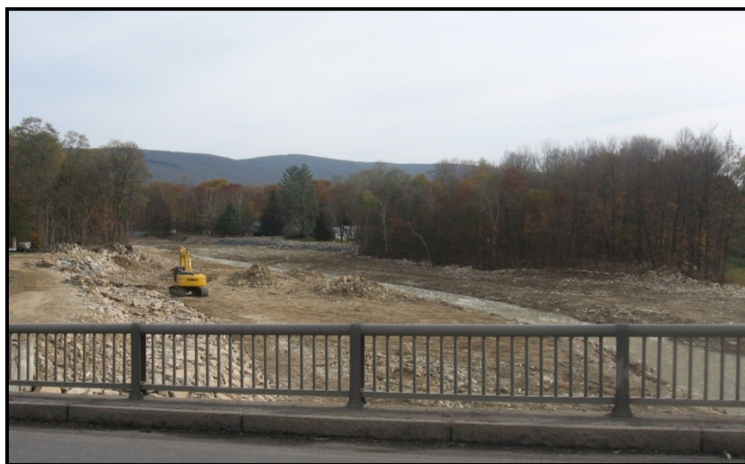
Figure 7: Construction of a new floodplain for the Roaring Branch, pre-Irene, above the Park Street Bridge in Bennington Vermont. (Kline, 2011)
