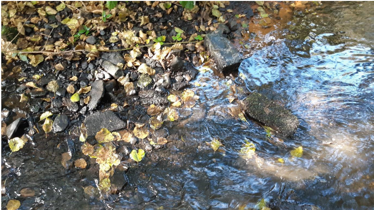
Figure 18: Gravel sized shale deposits - along with ochreous discharge and eroded brickwork.
