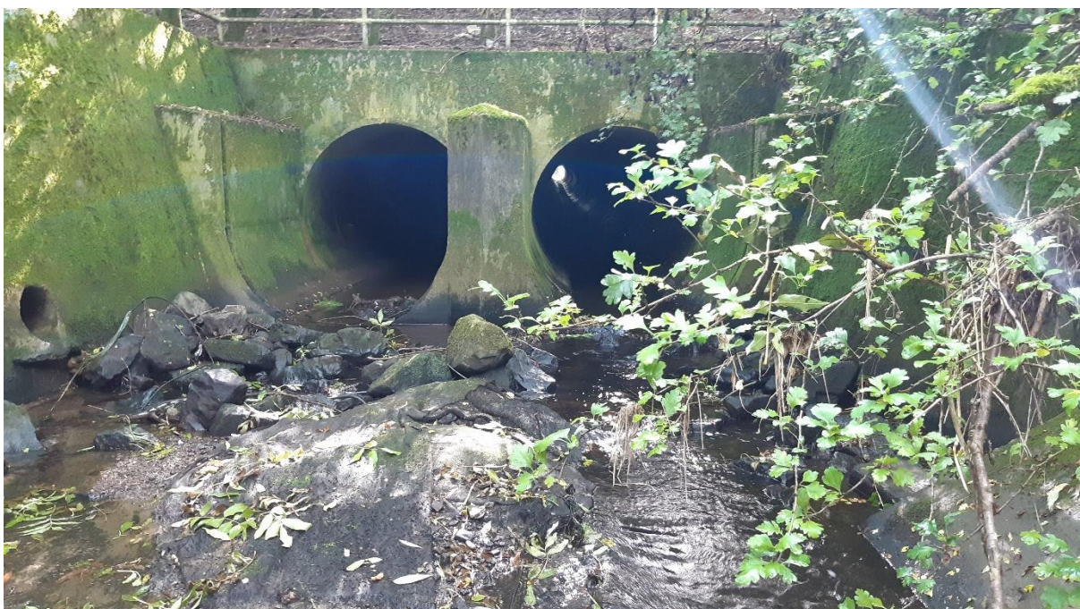
Figure 21: Twin pipe culvert running beneath the A617 at the top of Section 2 and setting the hydraulic limit for the downstream reach.
