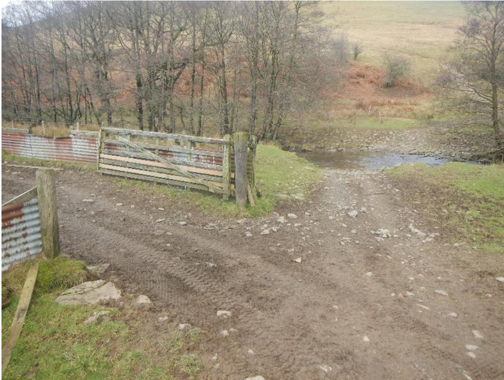
Figure 37. Track erosion and a likely source of surface runoff and fine sediment to the burn (55.185787, -3.084923).
