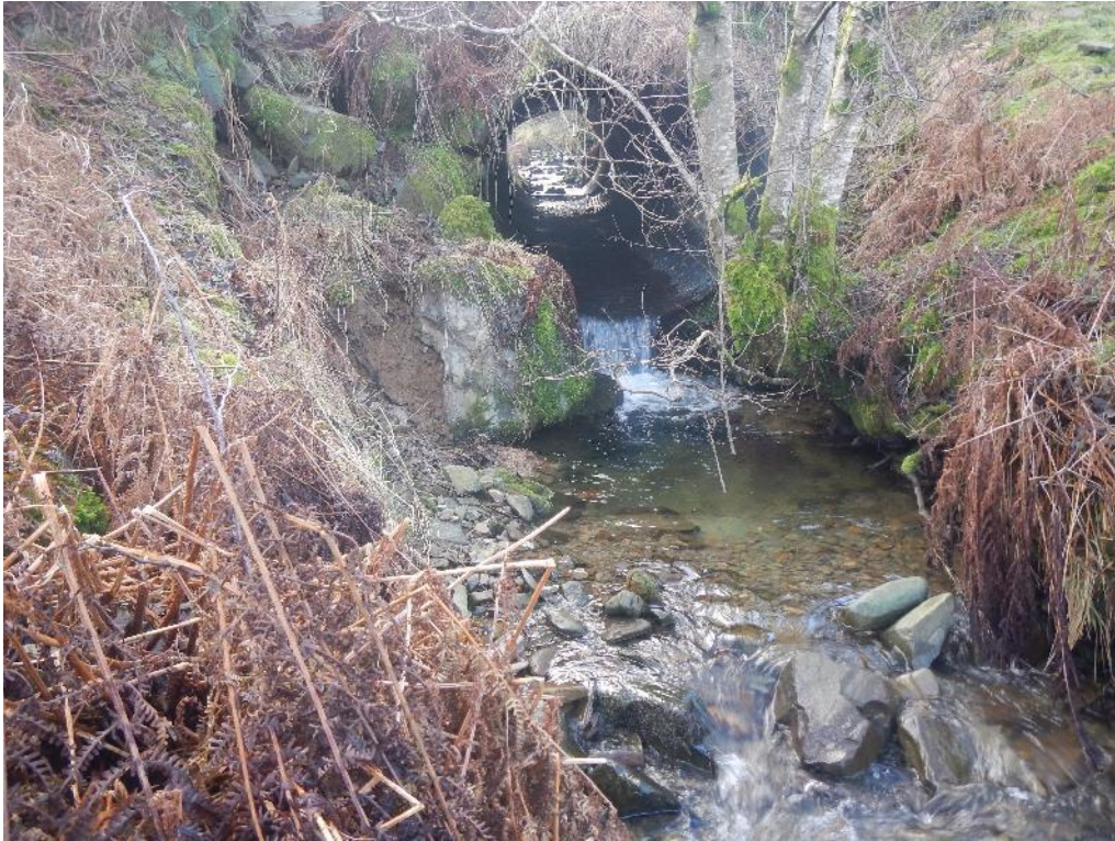
Figure 31. The potential of a viable spawning tributary is greatly reduced by the obstruction of a poorly installed, perched culvert (55.186822, -3.097292). While passable, this greatly reduces the opportunities for adult and juvenile salmonids to ascend.
