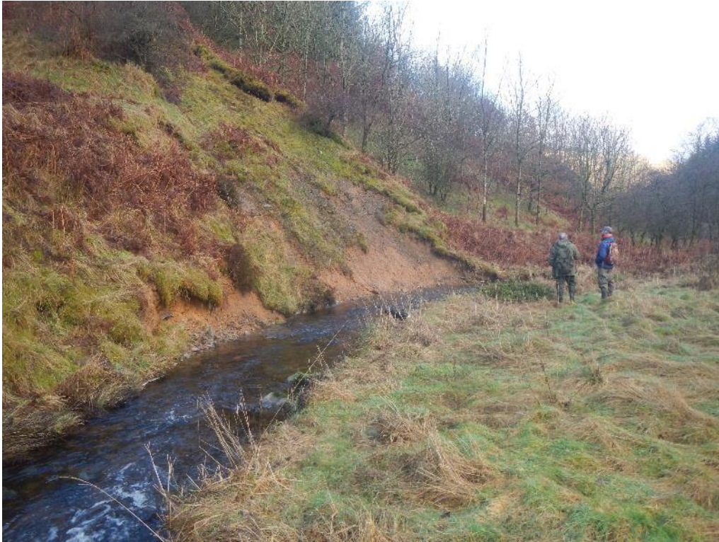
Figure 23. Without the protection of bankside tree roots, several of the sharper bends were subject to erosion and land-slipping (55.185703, -3.115677). It may be possible to install some Pinned Woody Material here on either bank, but it would require adequate anchoring to the bed and bank.
