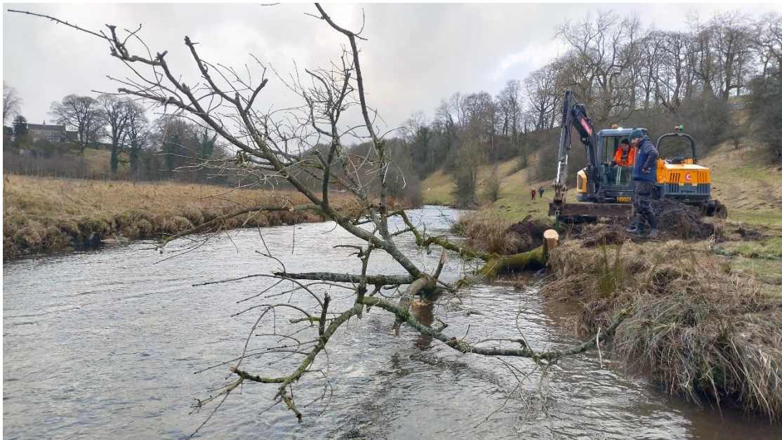
Fig 15. Felled ash being relocated and buried into the LB with available plant on an otherwise straightened and uniform reach.
