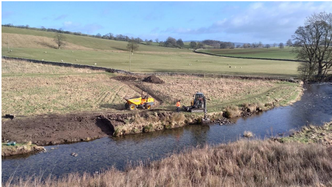
Fig 16. Lowering the LB artificial embankment to improve connectivity with a paleochannel in the floodplain, and returning any stone arising to the channel as a low bar to the LB.
