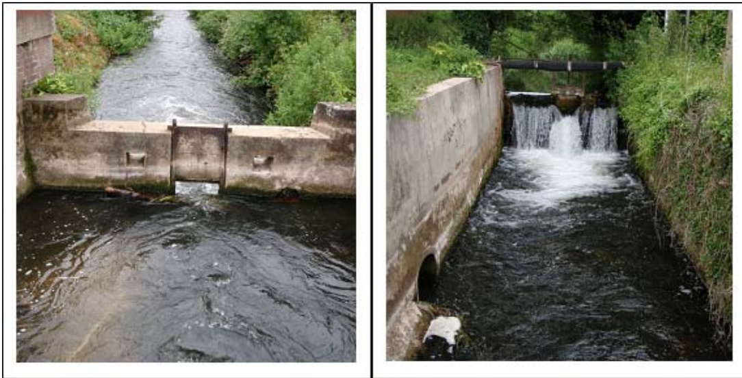
Figure 4.4 The sluice gate and vertical weir on the River Nar at Narborough, June 2008.
