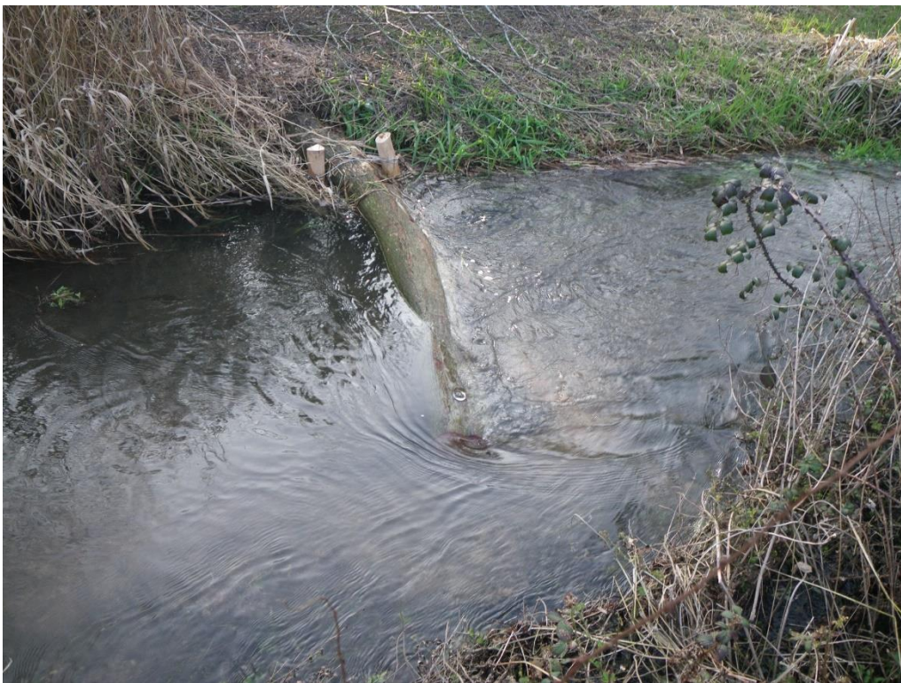
Figure 9 A log flow deflector set perpendicular to the flow and secured in place with chestnut posts and wire (bank end) and rebar pinned to the bed. Both overshoot and undershot flows will locally scour and clean gravel downstream of the structure.
