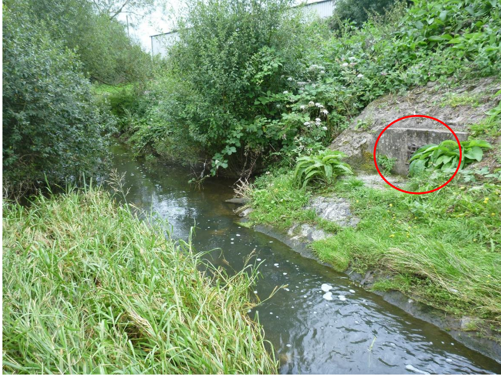
Photo 5 Downstream end of site (chainage 42.5m), end of artificial stone bank on RHB and flapped outfall (red circle).
