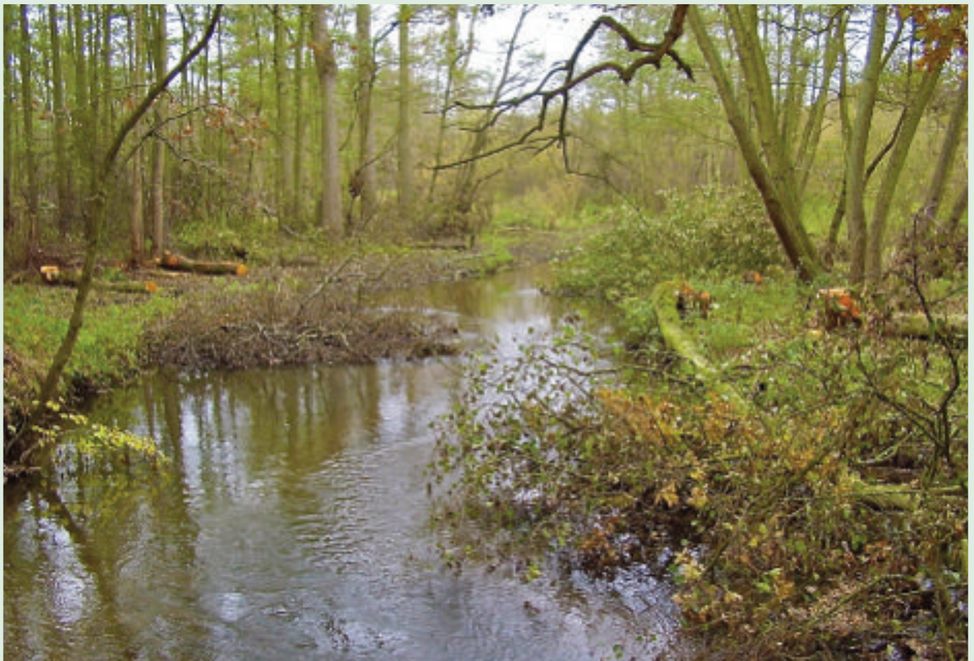
Blickling Fishing Club and National Trust - Installation of large woody debris into the River Bure upstream of Blickling Mill
