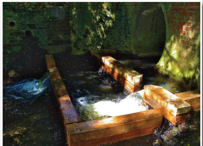
↑ A new box sections bolted to the concrete aprons will make upstream migration on the back of some extra water much easier this autumn
