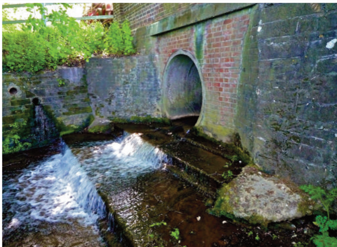
↑ The Batts culvert where sea trout used to pool up downstream, unable to make it up and through the culvert
