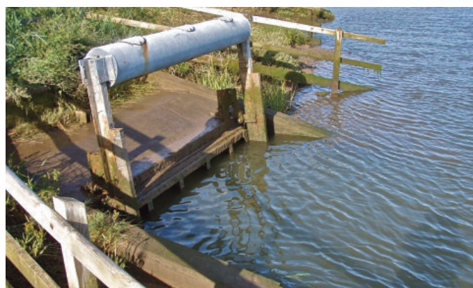
Photo: Tidal flap gate on the River Stiffkey – site of the new fish pass
